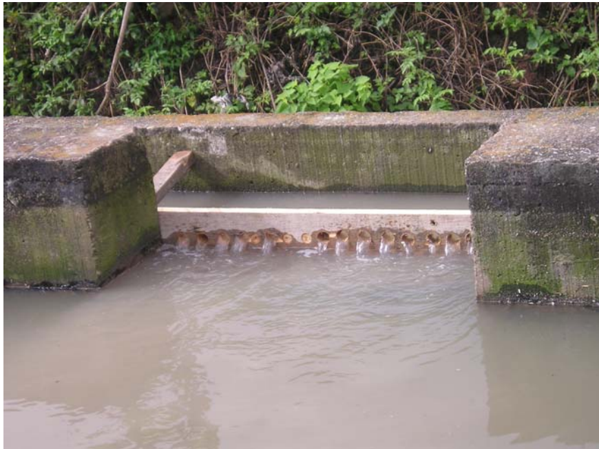
Figure 10 Control Gate for Flow Control in Imhoff Tank
